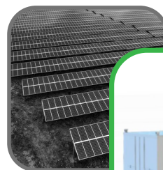
42+ acre solar farm
